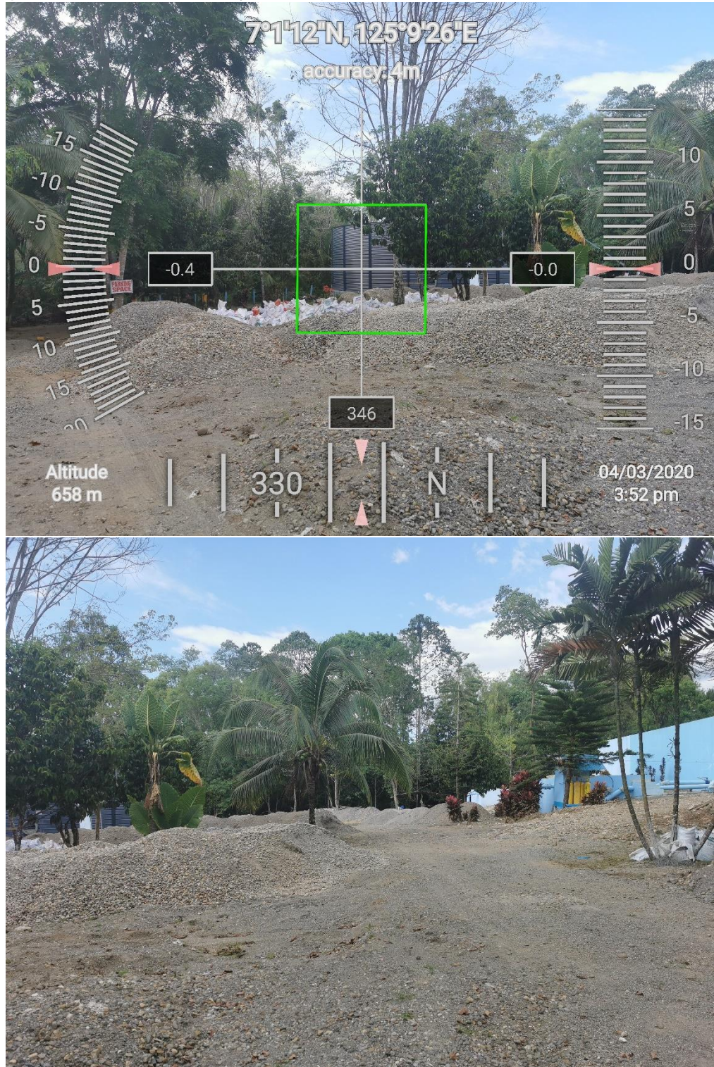
MKWD Lapaan Treatment Plant Facility, Brgy. Perez, Kidapawan City
